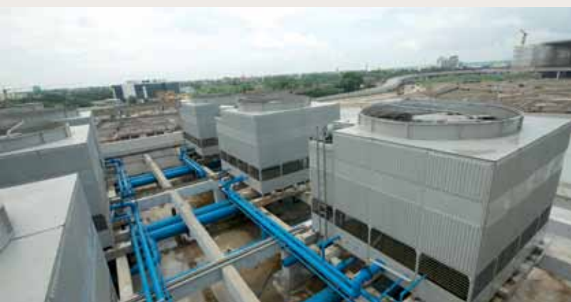
A panoramic spread of cooling towers.
