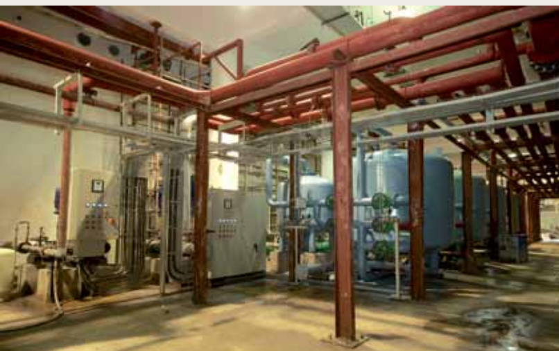
The water treatment plant yields 400 cu m per hour – the primary supply for wash-basins and drinking water.
