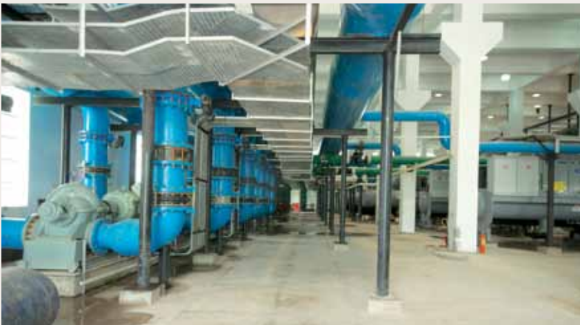
The mega-sized chiller plant room with its record-setting 12,000 TR capacity.
