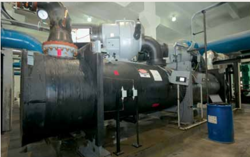
One of the four 2500TR centrifugal chillers.
